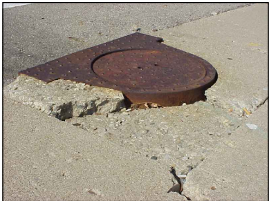
METAL OR OTHER PLATES, COVERS, OR GRATINGS THAT ARE NOT FLUSH (3/4 INCH OR MORE VERTICAL DIFFERENCE) WITH THE ADJOINING SIDEWALK SURFACE, ARE STRUCTURALLY UNSAFE, OR CAUSE A NUISANCE DUE TO SLIPPERY SURFACES ETC.
