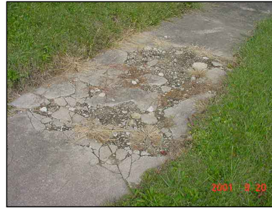
ANY SIDEWALK THAT IS DETERIORATED OR SHOWS SURFACE SPALLING, LEAVING IT VERY ROUGH, UNSAFE, OR WITH AGGREGATE PROTRUDING.
