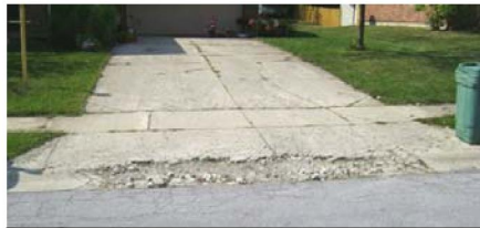
EXAMPLE: Gutter at Driveway
