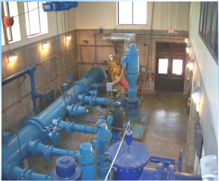
High Service Pumps
