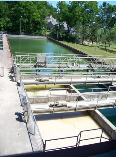
Pretreatment Flocculation & Settling
